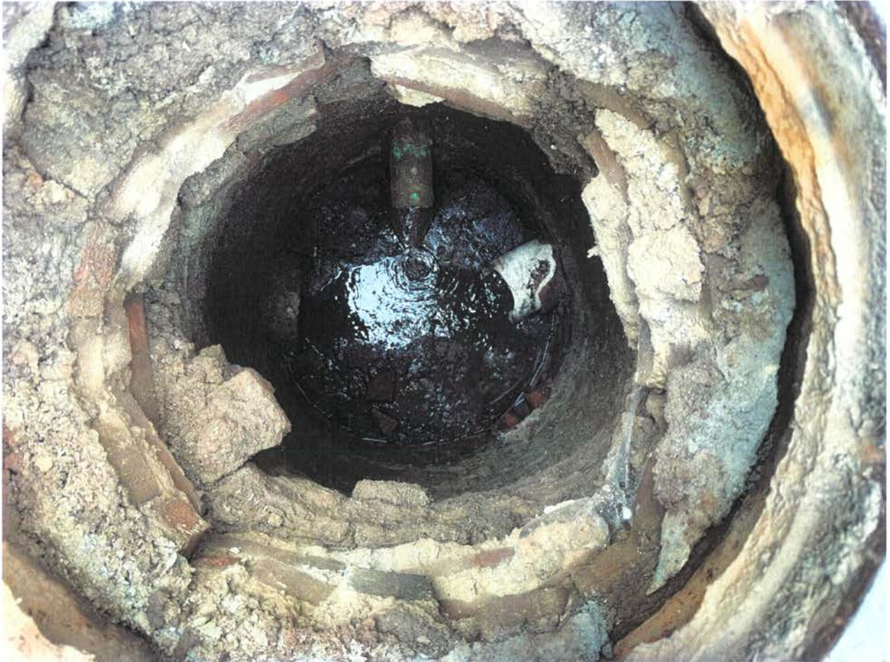
Kingsbury Sewer at Dennis Street
