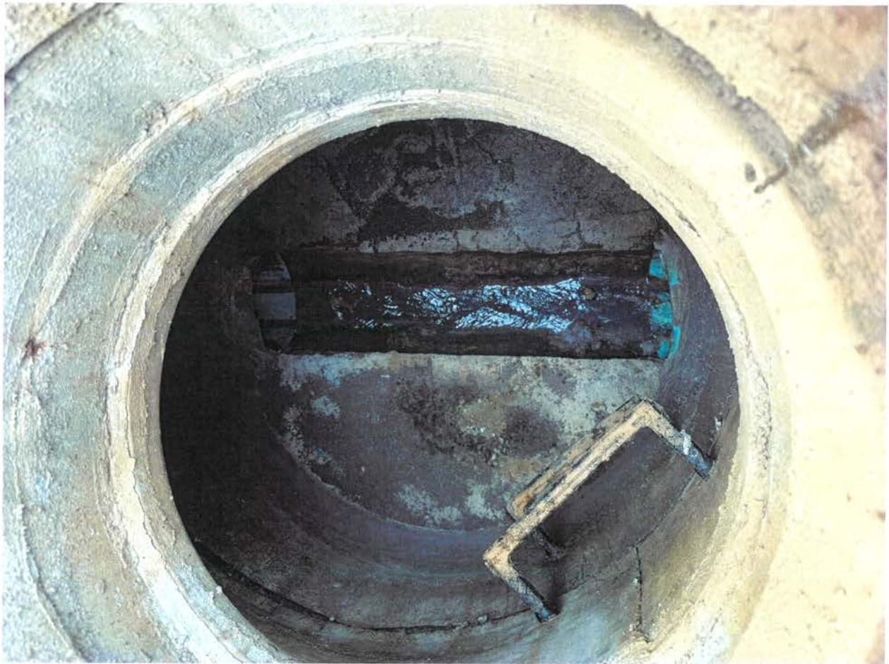
Autumn Street Sewer
