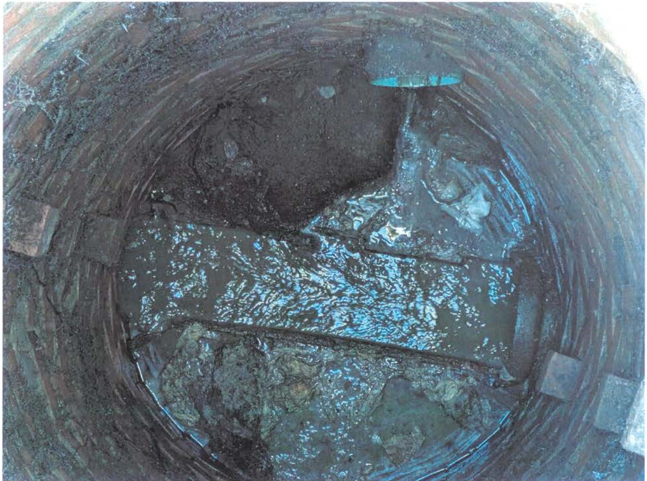
Cross-country sewer at Pleasant Street
